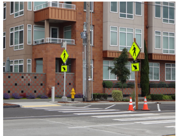
Solar-powered RRFBS can be mounted to metal or wooden signposts at crossings.
