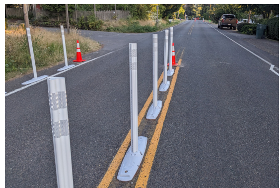
Flexible delineator posts installed along centerlines and edge lines encourage slower speeds.
