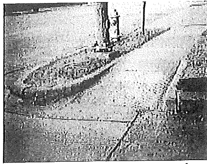
Figure 7-18. Detectable warnings at the bottom of curb ramps enhance access for people with vision impairments (Austin, Texas).
